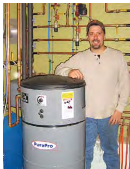
STEPHEN HAMMOND OF Refined Heating is pictured with a complete radiant heating system he recently installed.
